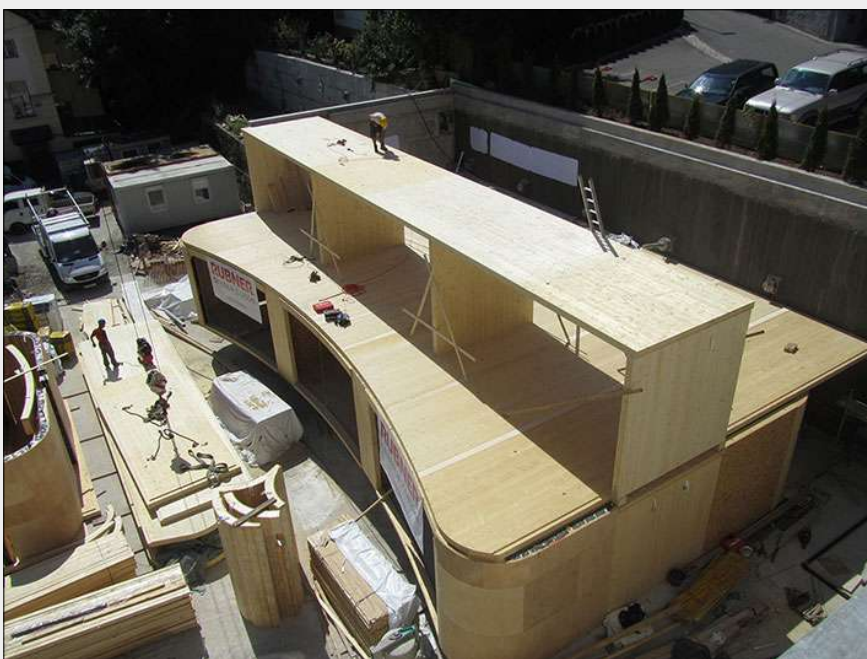
Fig. 6 - Prefabricated CLT elements are transported to the construction site and then assembled and erected manually: Waldorf School in Ljubljana, Slovenia built during 2009-2012.
