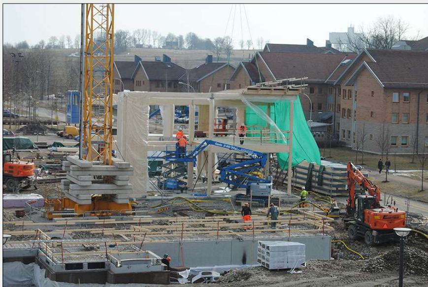
Fig. 5 - Glulam framework under erection for an educational building: “House N” at Linnaeus University in Växjö, Sweden (built in 2011).
